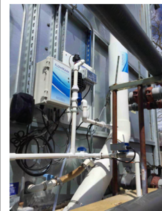
FlowMark Pulse Power Water Treatment System, Conductivity Meter & Blowdown Valve
