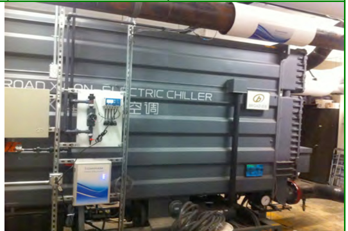
Chiller FlowMark Chemical-Free Electronic Water Treatment System with conductivity meter, probe and blow-down assembly.
